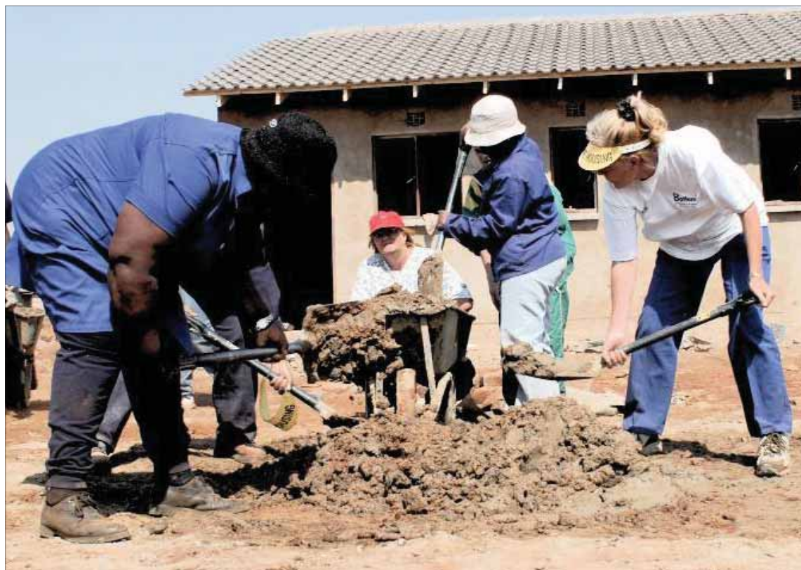
SENSE OF PURPOSE: Johanna Sello, Miems Coertzen, Basetsana Malema and Miranda Jooste dig the foundations for a house in Mamelodi. Having poor people construct their own homes will give them back their self-respect.
